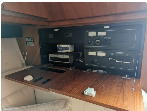
Tiara 3600 Open electrical panel
