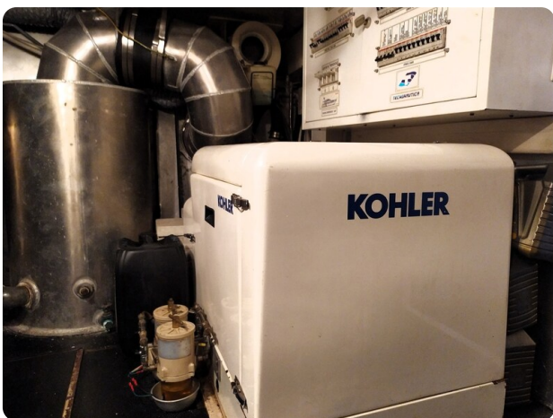
SANLORENZO SL 62 Generator
