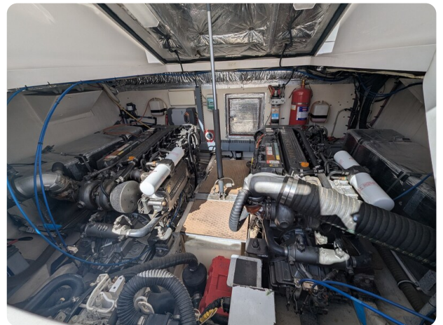
Luhrs 36 Open engine room
