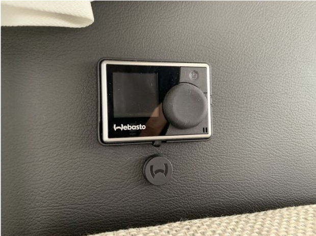
Jeanneau NC 37 twin diesel cruiser - Webasto heating controls
