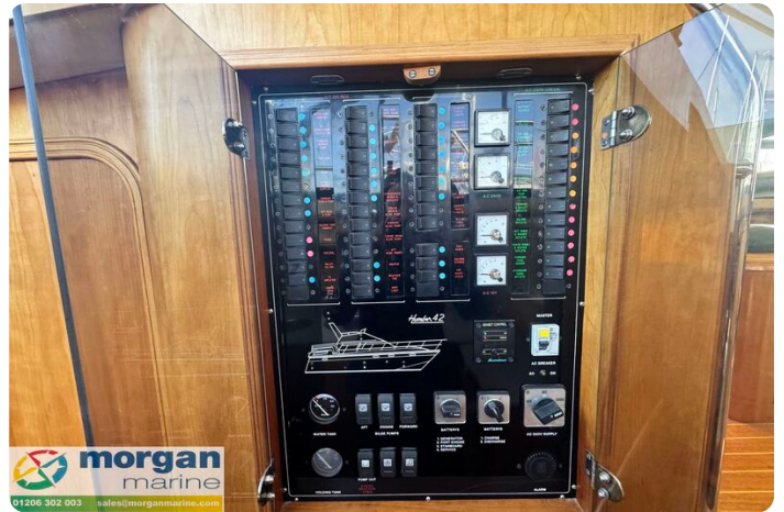
Humber 42 TSDY - isolators
