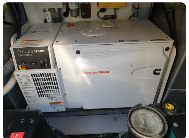
Beneteau MC5 generator
