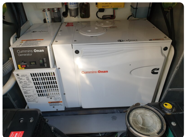
Beneteau MC5 generator
